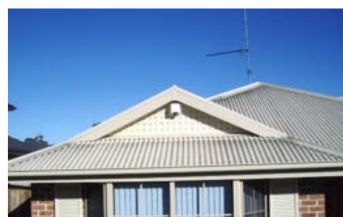
Figure 5. Roof made from COLORBOND® steel showing uniform coverage of fungus
